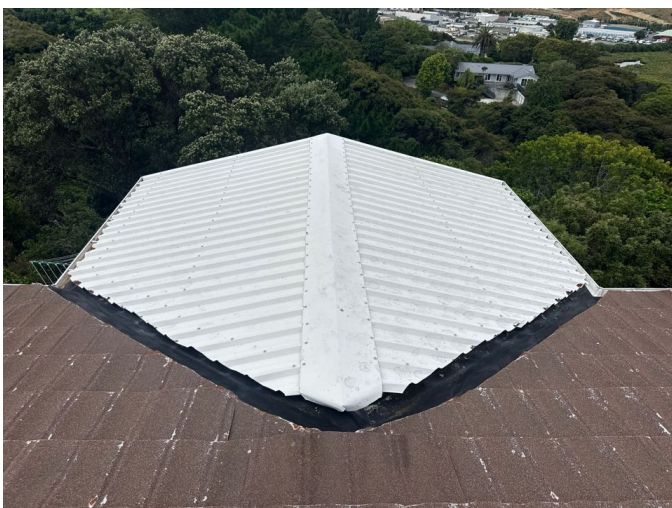
Rust to the edges of the steel roof. Rust treatment and paint touch up with slow the deterioration (recommended).
