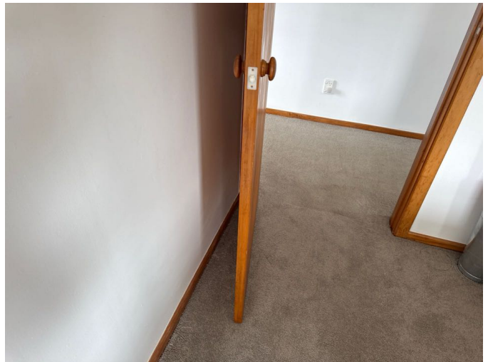
The internal doors are functioning well. Door stops should be installed where missing to prevent the risk of damage to the wall linings.
