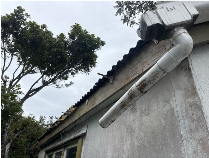
Spouting should be installed where missing
