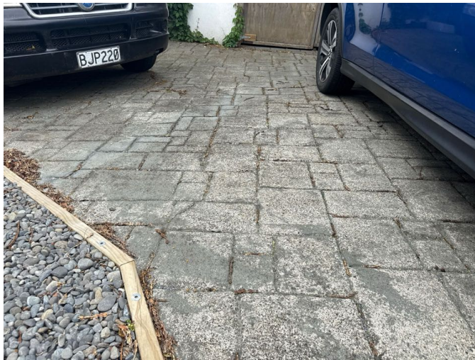
The driveway slopes towards the garage. Common and minor shrinkage cracking to the driveway noted.
