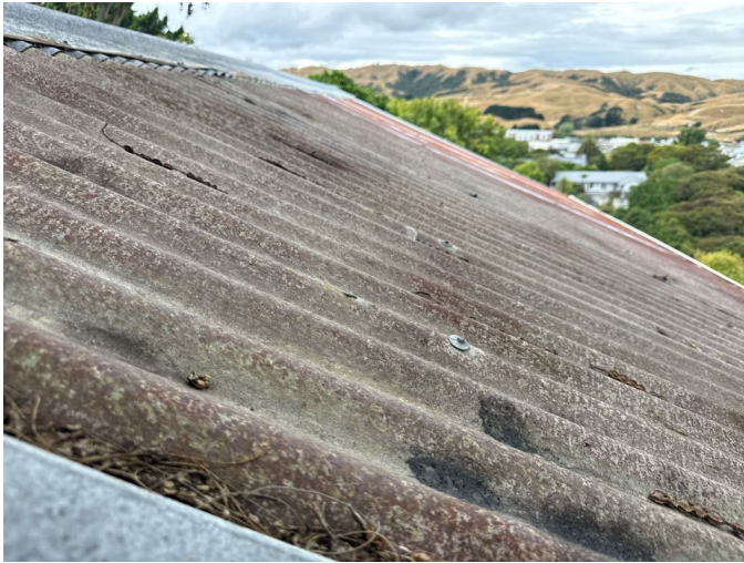
Rust deterioration to the roof. T.H.I.S recommends the roof be replaced in the short term.
