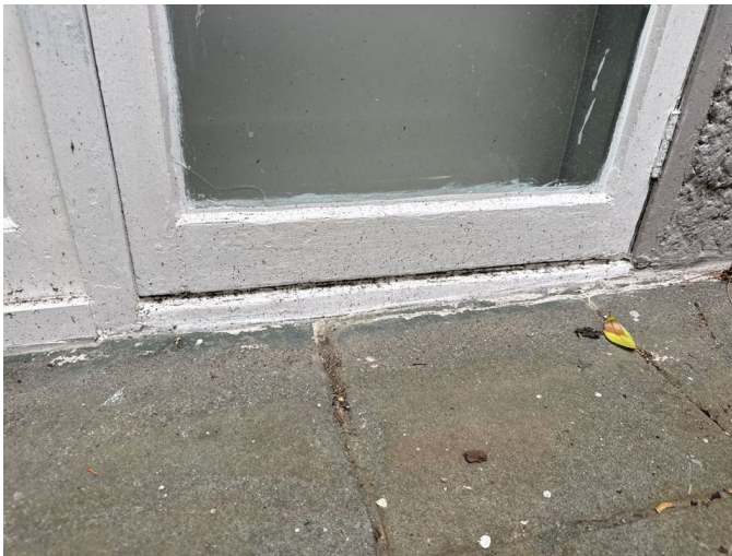
Timber in close contact with the ground is at risk of premature deterioration and must be kept thoroughly sealed. Paint improvements are recommended anywhere that surface wear is present.
