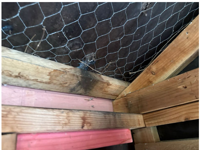
Moisture staining will need to be monitored until the roof is replaced
