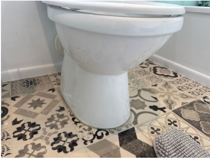
The base of the toilet is well sealed and secure. The toilet is in a functioning condition.
