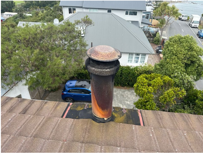
Age related wear to the steel flue. The waterproof membrane flashing appears to be secure, intact and effective.
