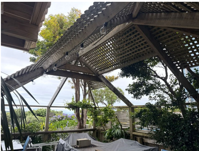
The timber pergola type roof was showing no evidence of significant deterioration
