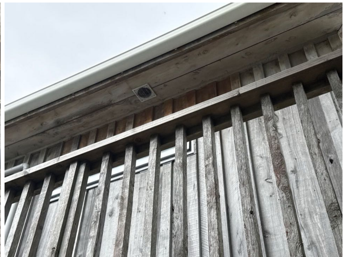
Extraction vents exit through the soffits
