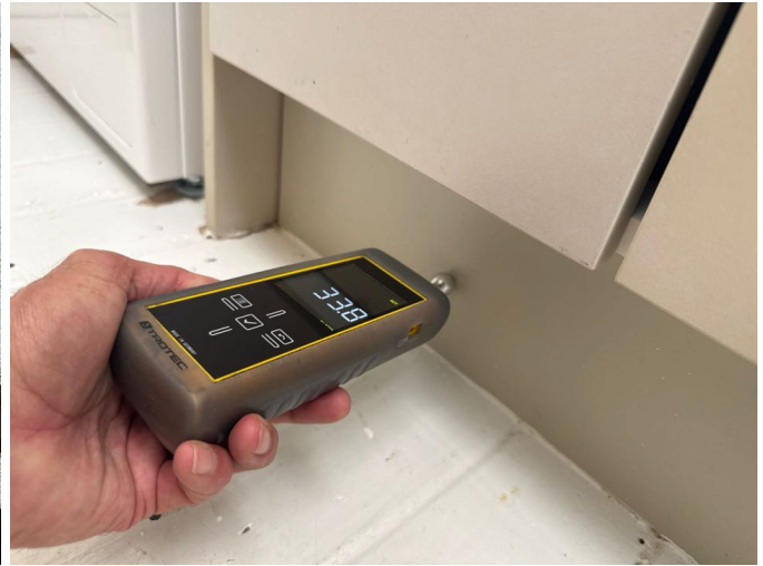
Moisture levels in the laundry were within the normal range at the time of inspection.
