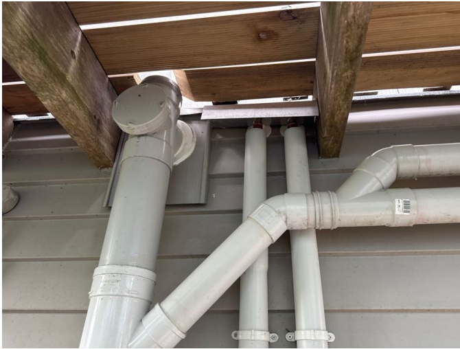
Cladding penetrations in general are a weather tightness risk area. Penetrations such as taps, screw fixings, gas or water pipes etc. A good seal must be maintained around all cladding penetrations over time to prevent issues. No evidence of failure could be found.
