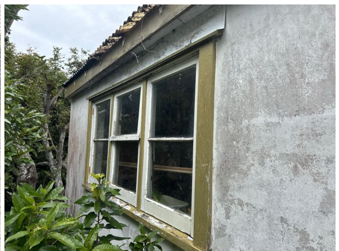
Deterioration to the timber joinery
