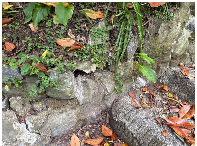
Deterioration to the original stone retaining wall on the steep east side. Retaining improvements are required where deterioration is present.
