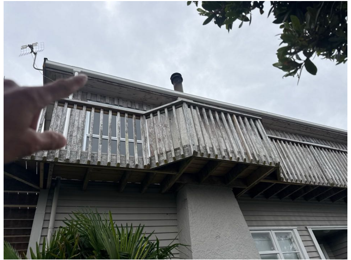
The cracked fascia board should be thoroughly sealed or the timber replaced
