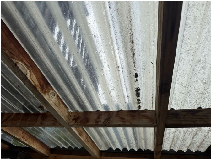
Moisture staining to the roof framing has likely been caused by condensation
