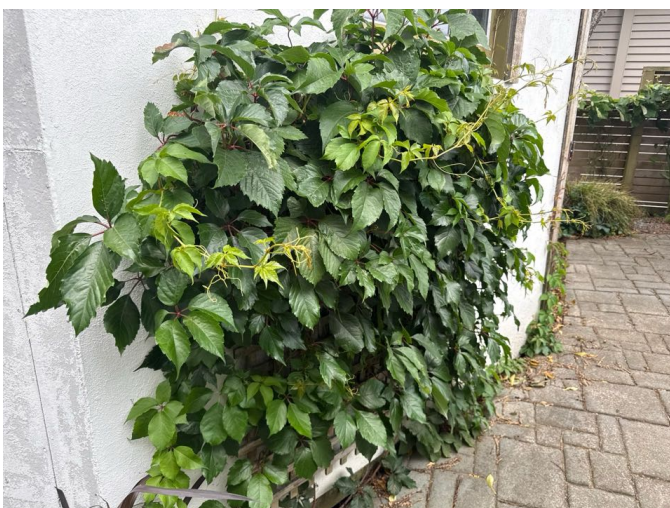
Vegetation should be removed from the cladding to prevent premature deterioration.
