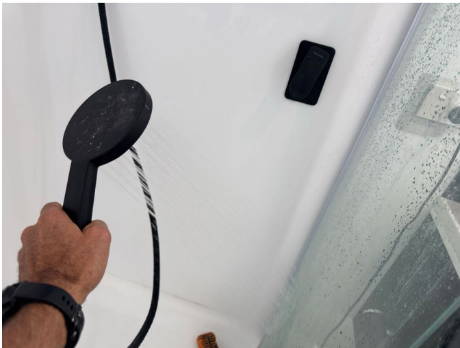
Good water pressure noted
