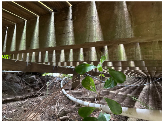
It was not practical to inspect all areas of the main structure due to the lack of room. There were no structural concerns sighted from the south side.
