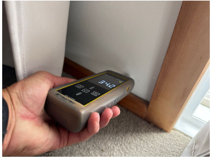
The moisture levels to the external walls were within the normal range
