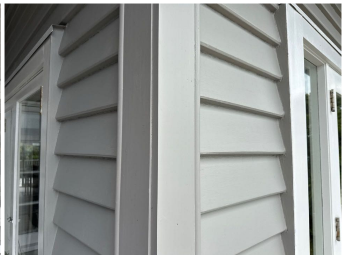
Timber box corner and scribe detail to the external corners. Box corners protect the external weatherboard joins from deterioration and is a second layer of weather protection. Well installed and sealed throughout.
