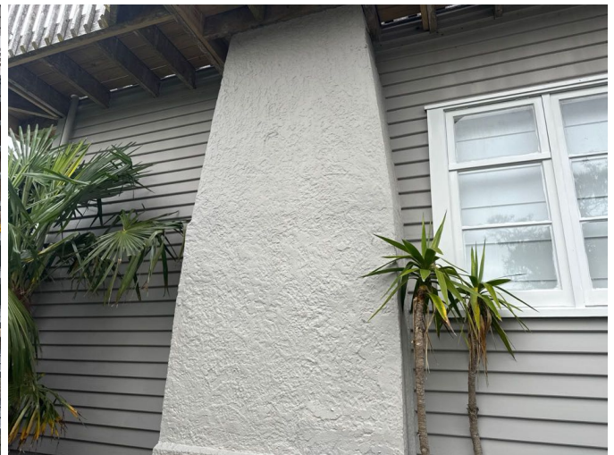
There was no evidence of damage to the concrete chimney base at the time of the inspection. The cladding junctions are effectively sealed.
