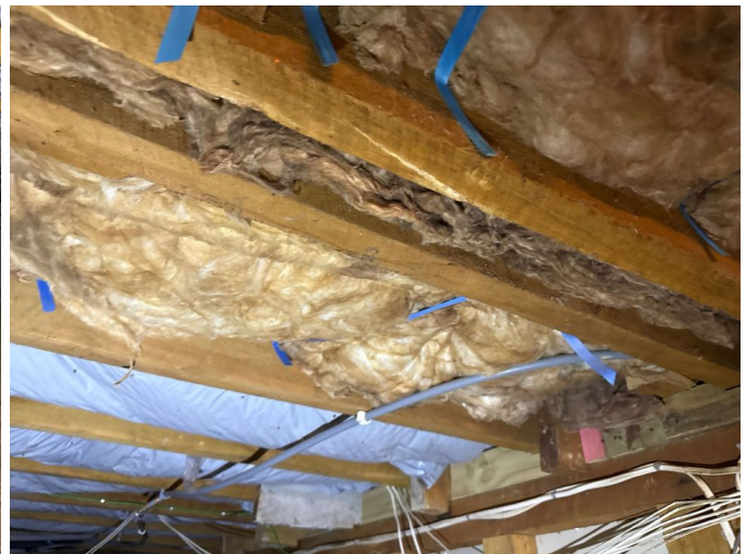
Batt type insulation installed in the sub floor. There was no labelling present to indicate the R-Value of the material. The thermal resistance rating or R-Value is the measure used most commonly in the building and construction industry to determine a material's ability to resist the transfer of heat. The higher the R-Value the better thermal resistance the product will provide.
