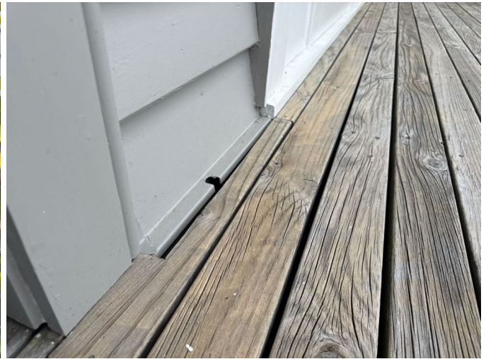
Clearance gap and cladding junction noted. The gap will allow water to drain away.
