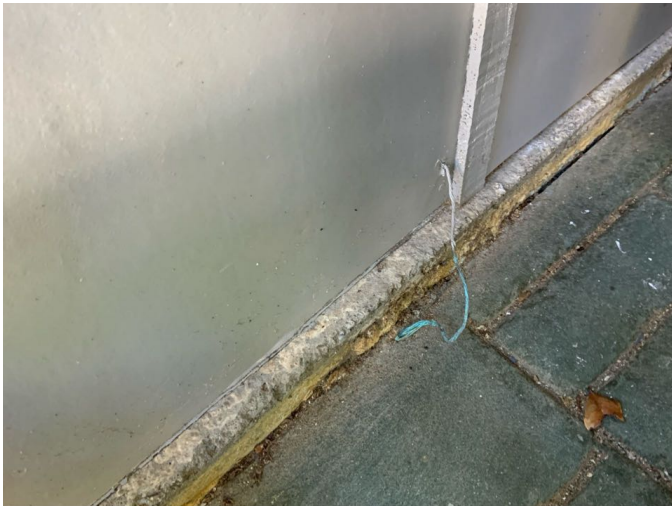
Earth wire under the back stairs. No rod sighted.
