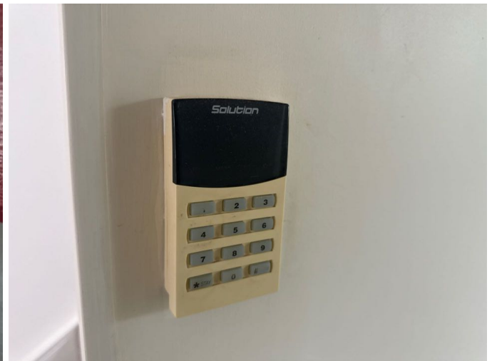
The alarm system is not functioning
