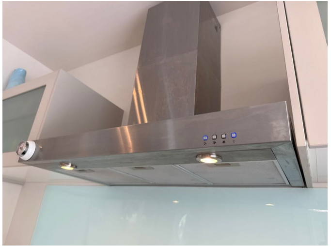
The range hood extraction unit is functioning
