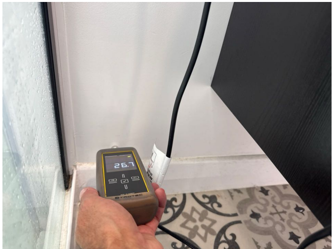
The common fail areas of the shower and plumbed areas were checked for elevated moisture. Moisture levels were within the normal range.
