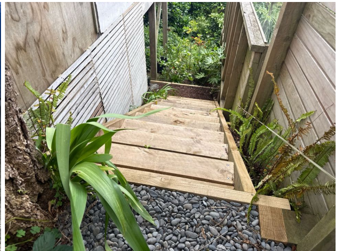
The timber stairs down the south side of the garage are solid and secure
