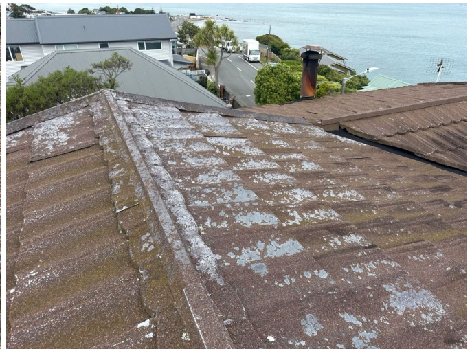
Surface wear to the chip coating
