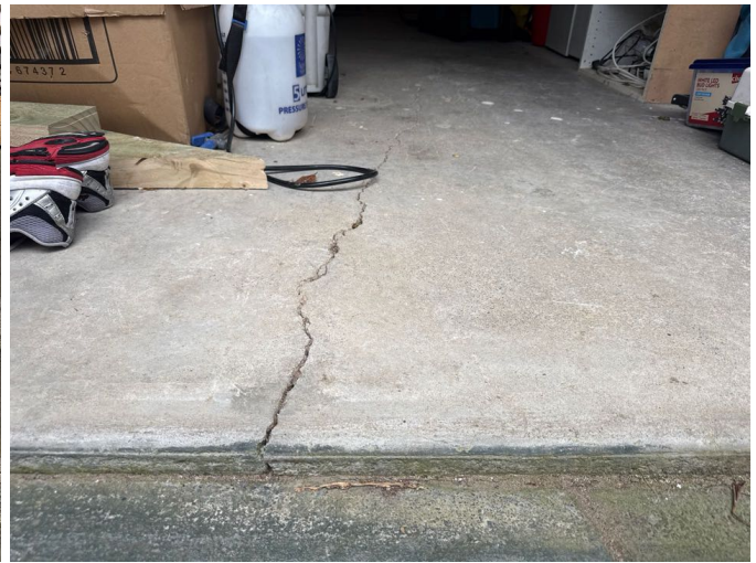
Common shrinkage cracking to the garage slab. This is not a structural concern and is commonly caused during the curing stage of the concrete hardening process.
