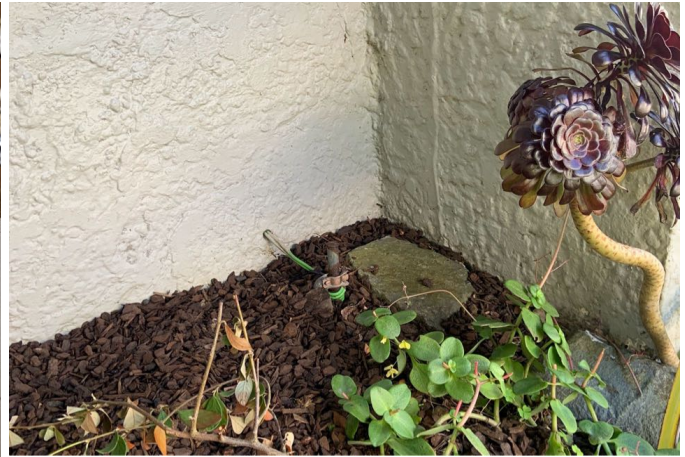
Left side of the chimney. The electrical earth rod provides a safe path for fault currents to dissipate into the ground, helping protect people and equipment from electric shock and reducing the risk of damage during faults or lightning strikes. An earth loop test should be completed by a registered electrician to determine the earths effectiveness.
