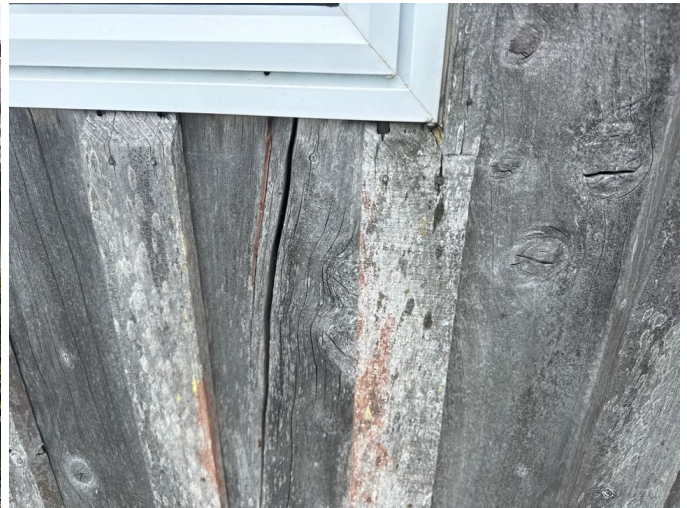
The cracked weatherboards are at risk of rot damage and water ingress issues. Thorough waterproofing improvements are required or the boards replaced.
