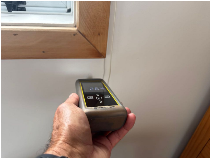
The moisture levels to the external walls were within the normal range
