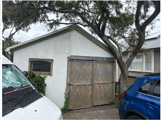
General age related wear to the garage. The manually operated timber doors are functional.
