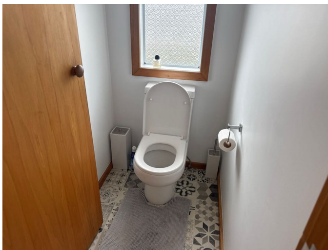
The base of the toilet is well sealed and is secure. The toilet is in a functioning condition.
