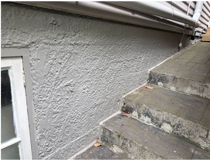
The concrete ring foundation is in a typical condition for the age. No sign of cracking or significant stress.
