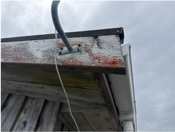
The unsealed barge boards and fascia are in an average overall condition
