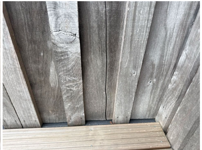
Cracks at various locations
