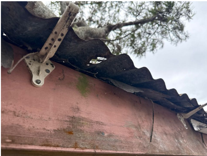
Another example of the rust deterioration to the roof
