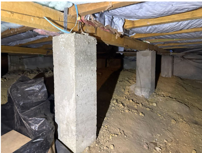
The concrete piles are solid at the time of inspection. Galvanised wire connects the bearers to the piles and anchors the structure to the ground.
