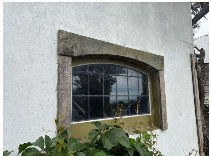
No head flashing over the window. The head must be kept well sealed to prevent the risk of weather tightness issues. Head flashings should be installed to reduce the risk.
