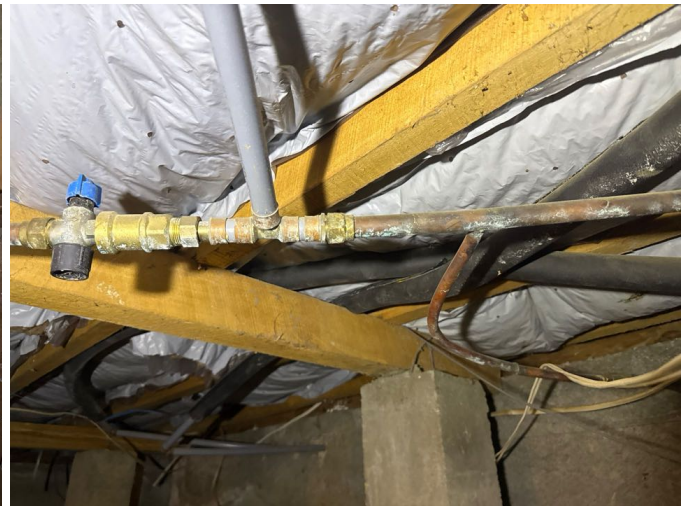
Only Buteline and Copper pipes sighted during the inspection
