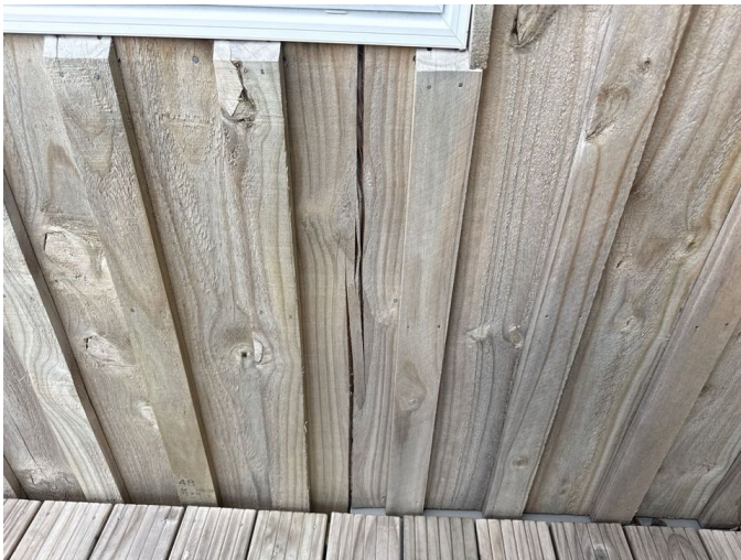
Significant crack to the new cladding. Waterproofing or replacement recommended.
