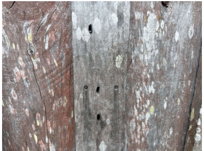
Example. Any holes in the cladding or battens should be sealed.
