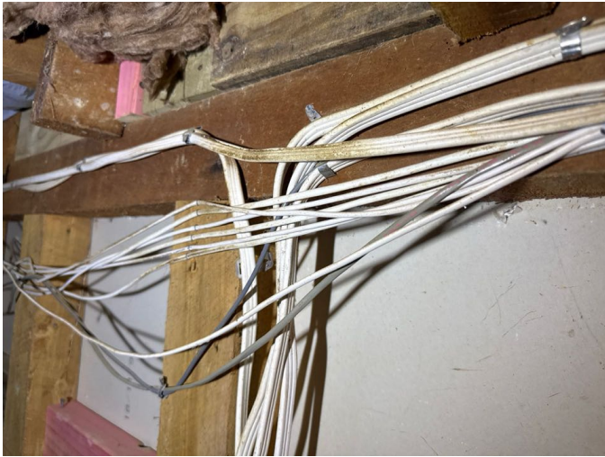
Only modern TPS wiring sighted during the inspection. There was no earth rod sighted during the inspection.
