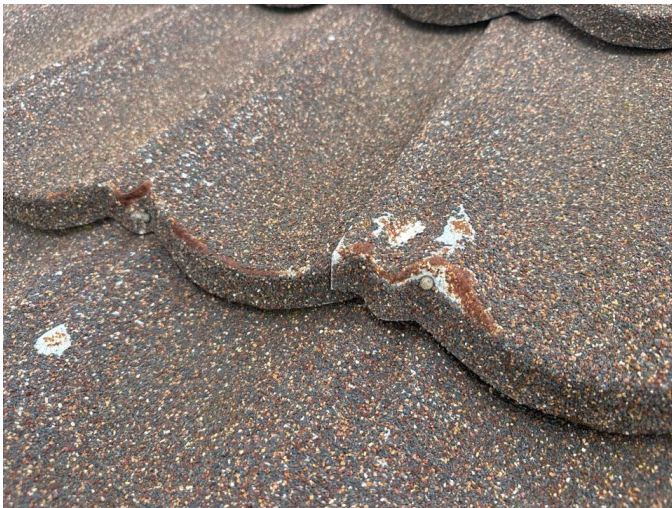
Example. Rust to the tiles at various locations.
