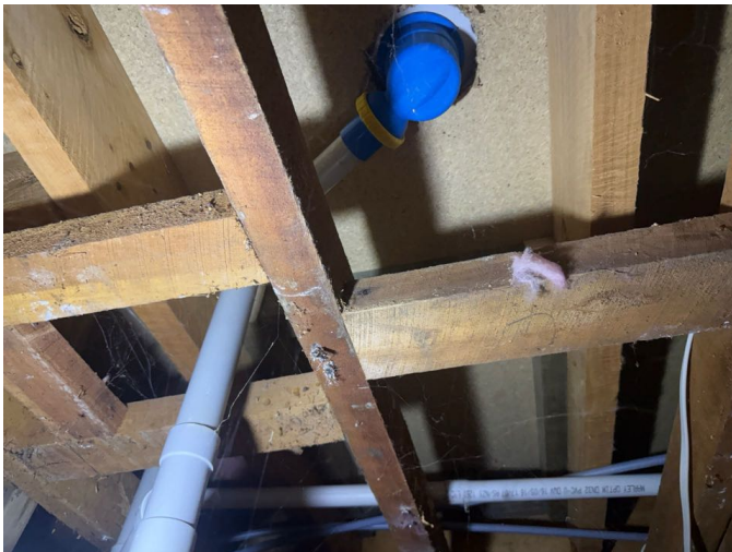
Example. There was no evidence of current leaks under the plumbed areas.
