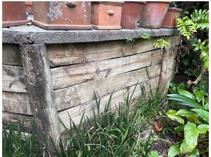
Age related wear to the timber retaining walls which will need to be monitored. These are still effective.
