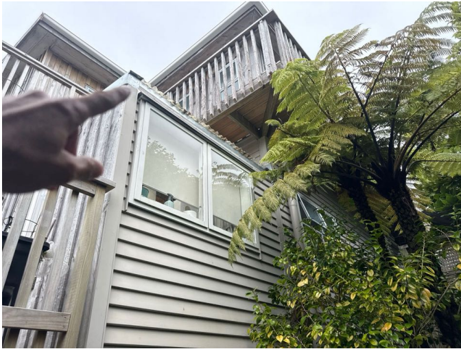
There is no spouting beneath the extended section. This has not caused any significant issues to date.
