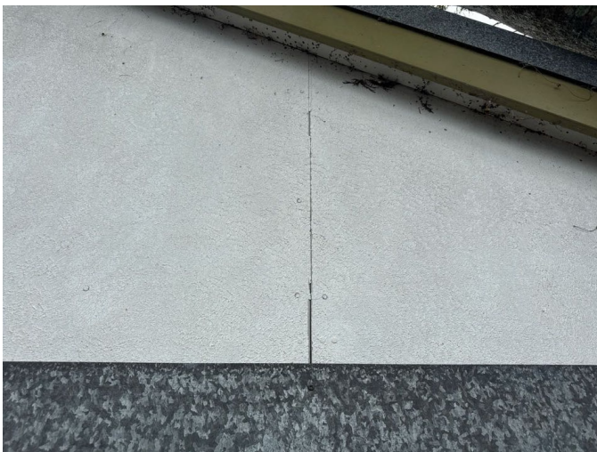
Example. Gaps in the cladding are a potential weather tightness risk and should be thoroughly sealed. A comprehensive paint upgrade is required to the exterior.
