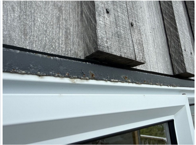
Some of the homes head flashings have superficial corrosion. This will get worse if left and requires the corrosion to be removed before sealing with rust converter and painting. Risk of water ingress issues if left to deteriorate.
